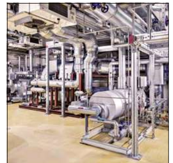
30 District steam heating of a dairy plant Technology/IT
