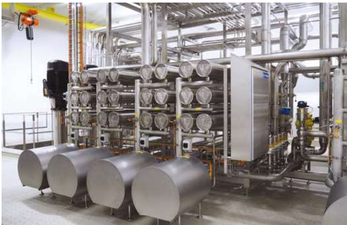
The heart of the Fonterra project is a new ALPMA RO HighTS plant (photo: IDM)
