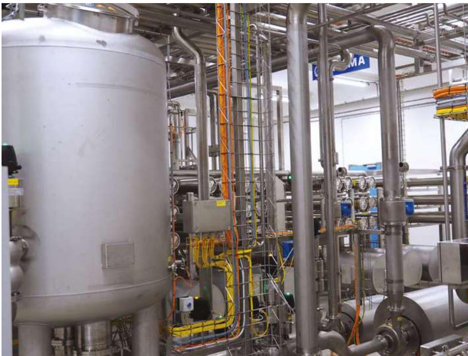
The turnkey project supplied by ALPMA/LTH encompassed not only the RO plant, but also automation (for which long-term partner Beenen was subcontracted) and a CIP solution (photo: IDM)
